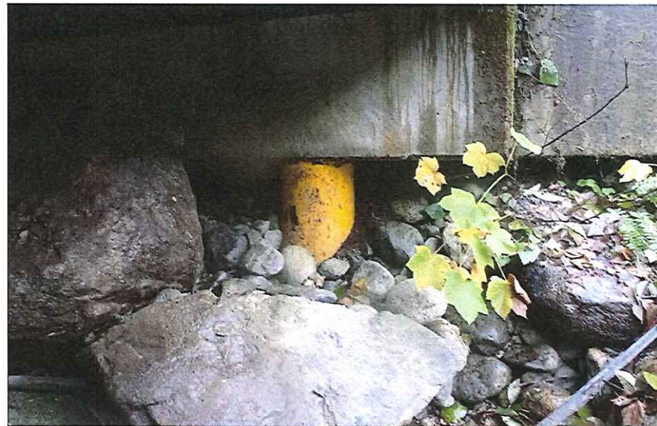
CK2417 Left Abutment post with rust starting
